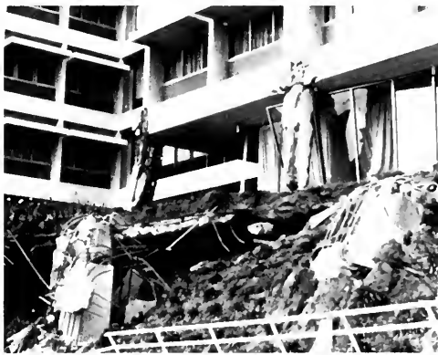
Photo 32. Column punched through the roof slab supporting a landscaped area at the first floor level.
